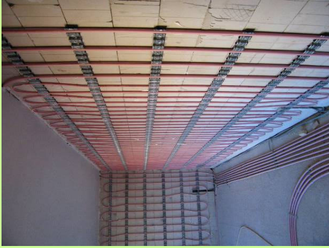
Silicate block wall and surface heating ductwork.
