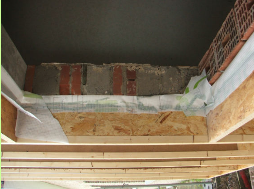
Timber frame construction fixed to the existing wall. The originally wall was erected with concrete blocks, but during the retrofit and the adaptation of the windows some clay tile blocks were build in.
