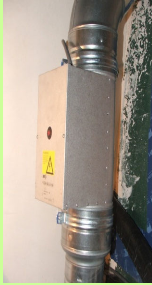
An electrical resistance for post heating the living areas.
