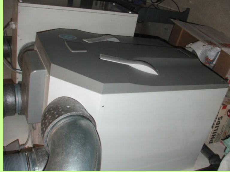
Mechanical ventilation unit.
