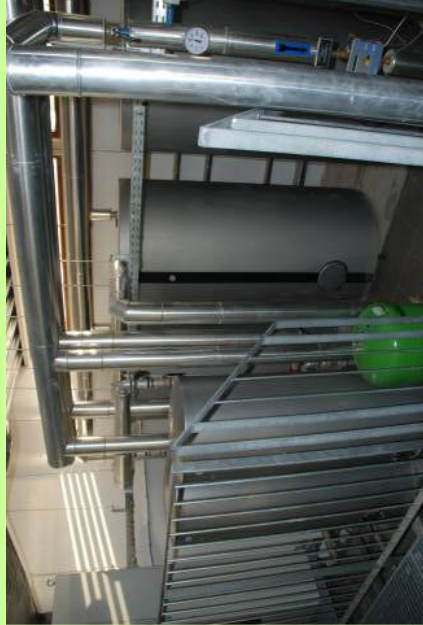
The 2 3000l buffer tanks in front, and the 3 1000l buffer tanks in the back.
