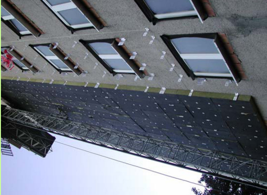
Mineral wool insulation being installed on the existing concrete walls of the north façade.
