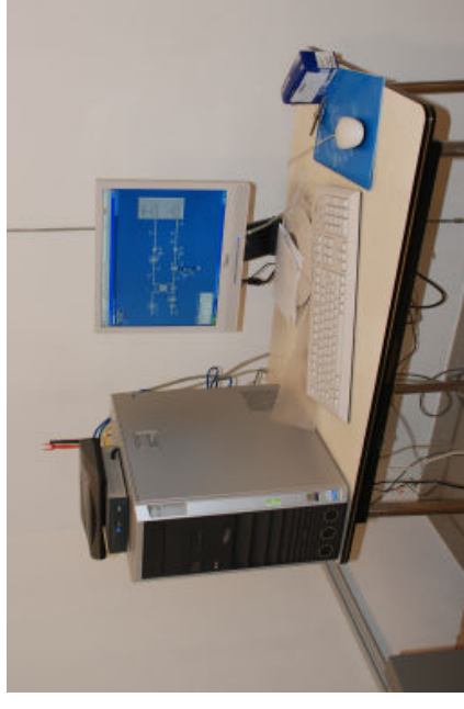
The central monitoring system for the buildings Zonneveld and Sterrenveld.
